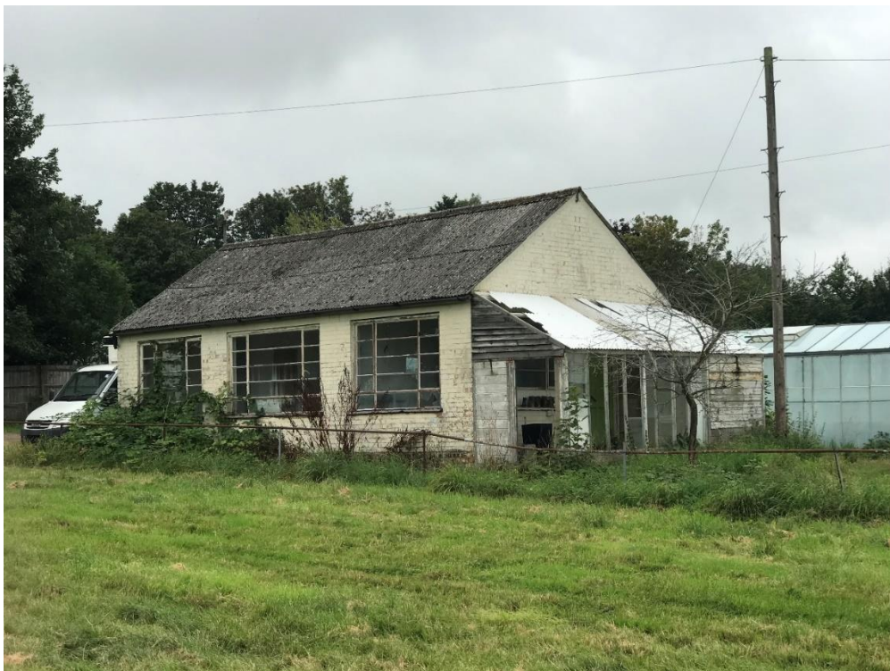
Photo 16: View of a Dilapidated house at the site
