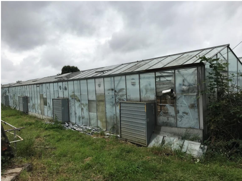
Photo 6: View of the greenhouse (unsafe to use) at the rear of the site
