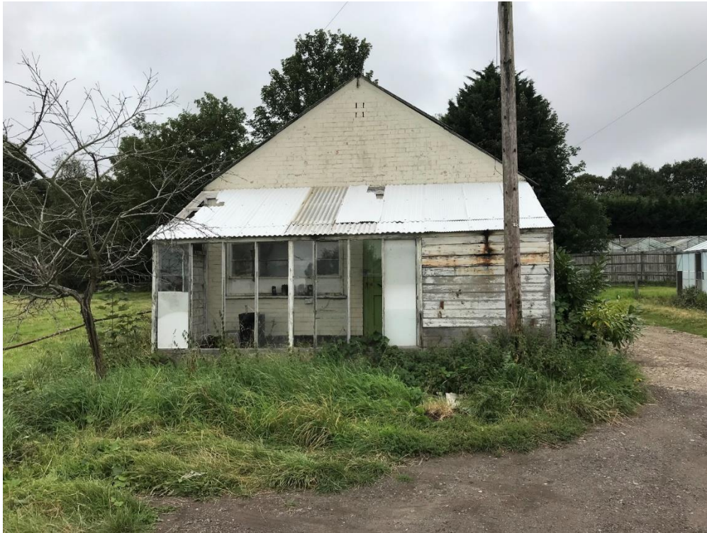
Photo 17: View of a Dilapidated house at the site
