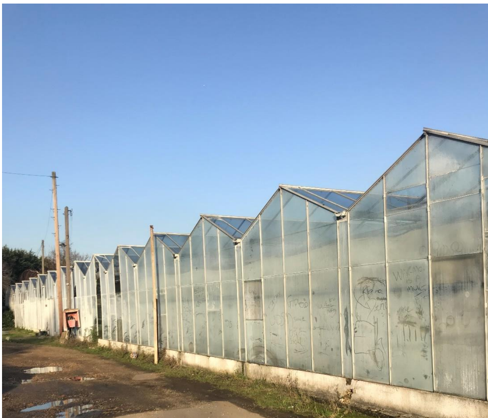
Photo 4: View of the greenhouse (unsafe to use) at the rear of the site
