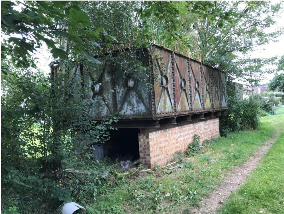
Photo 23: View of derelict water tank at the site
